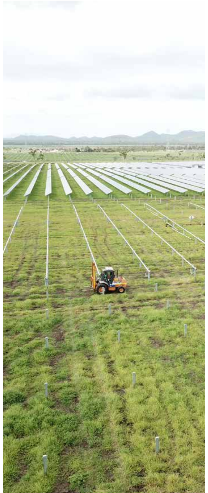
Whitsunday Solar Farm. Image Courtesy: Edify Energy
