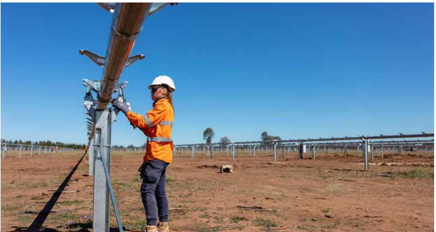
Western Downs Green Power Hub. Image Courtesy: Queensland Government
