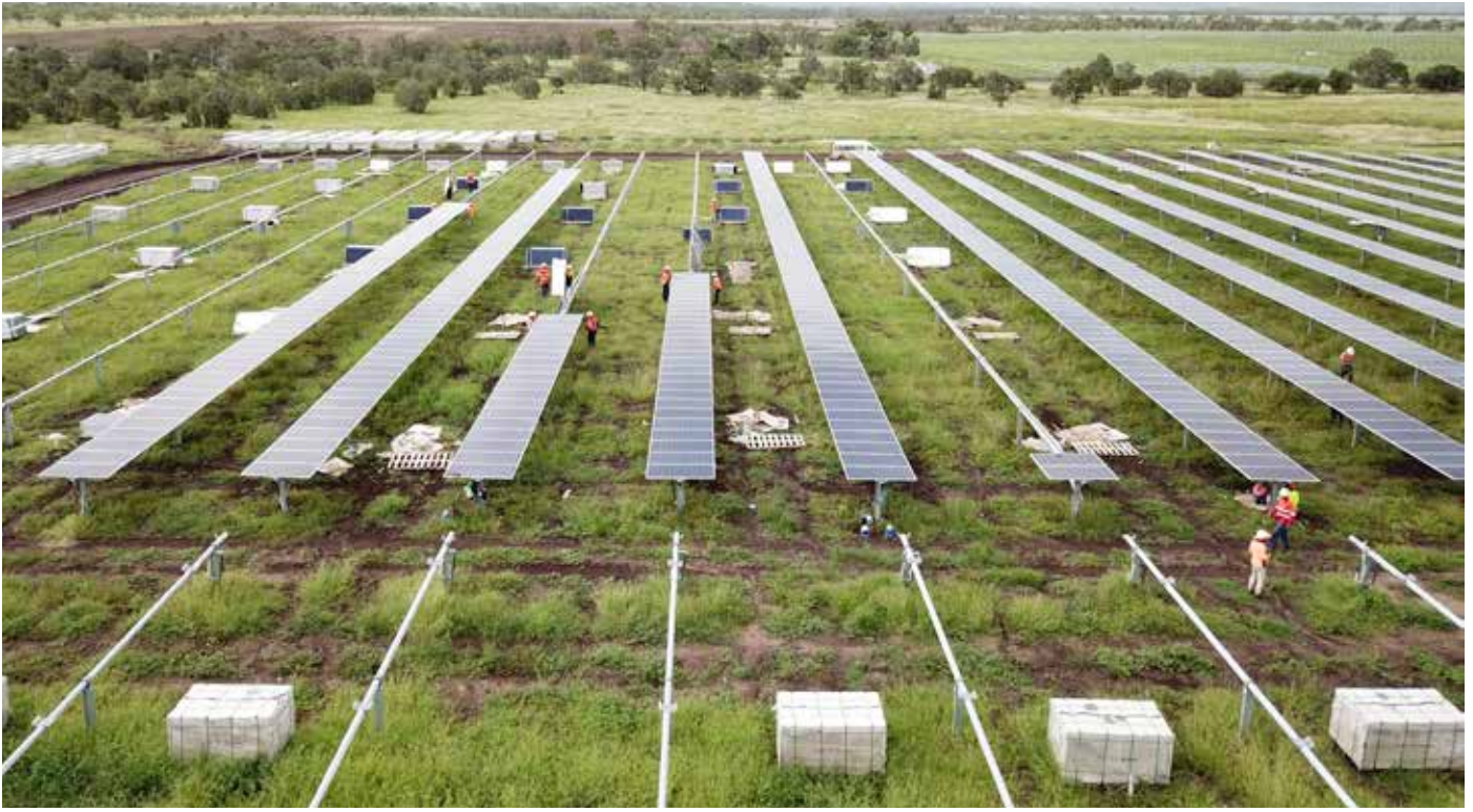
Whitsunday Solar Farm. Image Courtesy: Edify Energy
