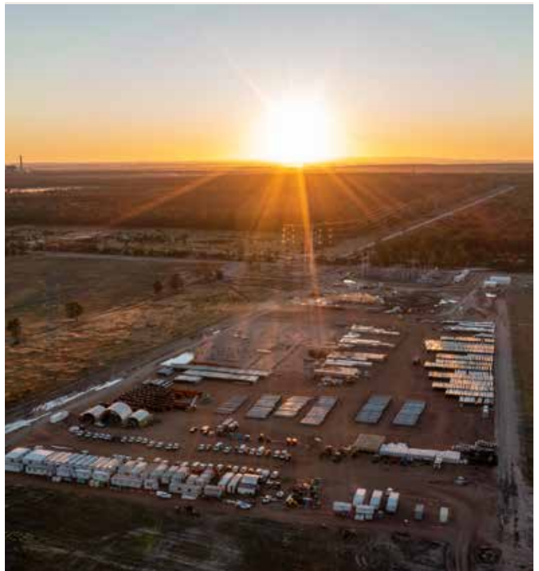
Western Downs Green Power Hub. Image Courtesy: Queensland Government
