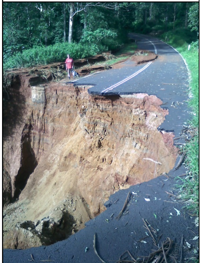
Many roads and infrastructure—including this road in the Lockyer Valley—were severely damaged in the floods.
